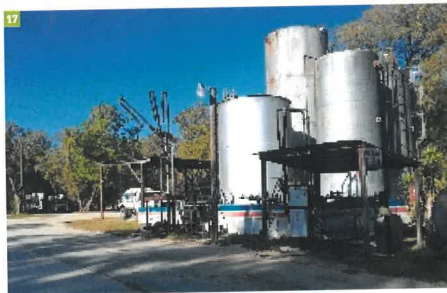
(17) A top-loading fuel dock and tanks.
