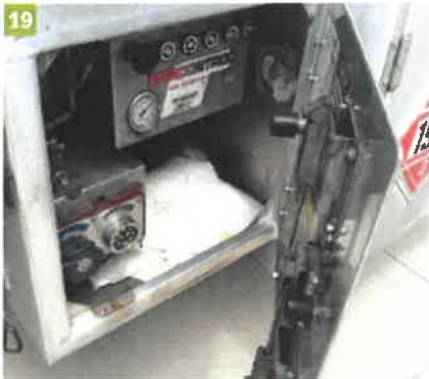
(18) Manual belly valve controls on a four-compartment tanker. (19) Pneumatic belly valve controls on a five-compartment tanker. Note the two black plungers on the door that release the corresponding actuators when the door is opened. The actuators simultaneously lock the trailer brakes and open the top vapor valves. Also note the thermistor/optic plugs in the lower left for static control at the loading rack.
