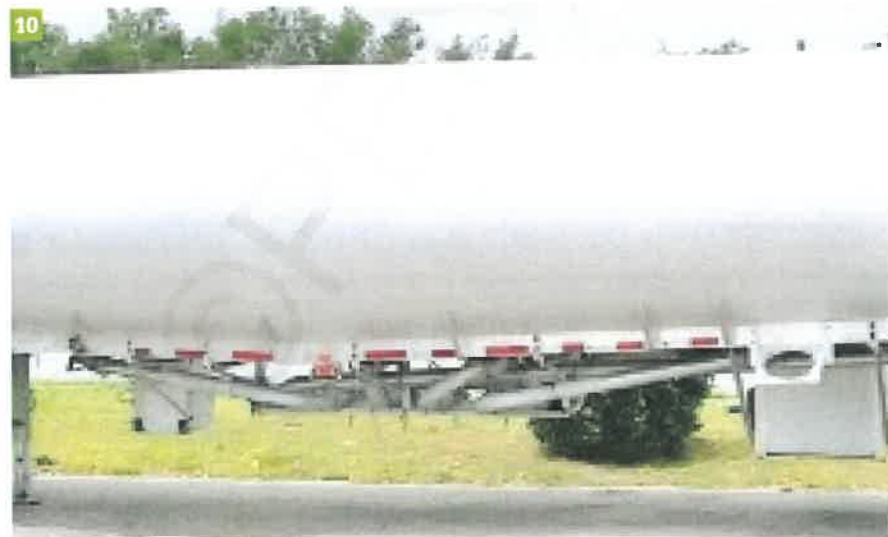
(10) The belly piping (wet lines) of a four-compartment tanker trailer.
